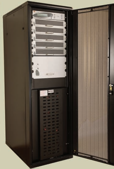
RM 50KVA Complete: POWER+ FS 10-50KVA ; MMBS; Battery Cabinet 64x 20Ah in Rack
